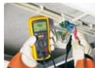
Wiring test in a small distribution box – all in one spot
