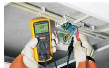
Wiring test in a small distribution box – all in one spot
